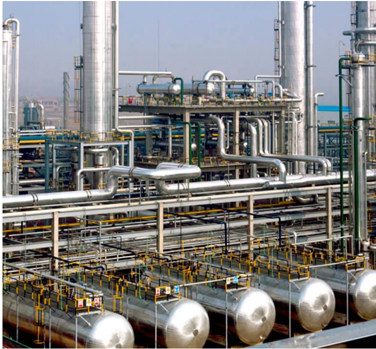
Figure 2 – Chemical processing plant balance of plant components are commonly built from stainless steel [8].
